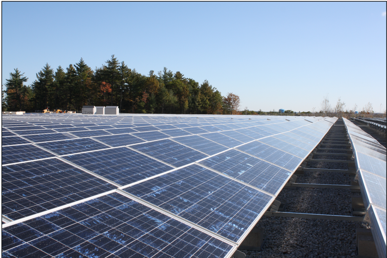
Westford Solar Park, photo courtesy of EEA
